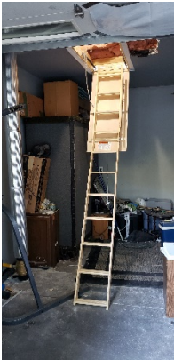
12101 Brewster garage attic ladder
