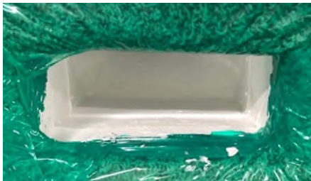
34480 Capitol coated duct work
