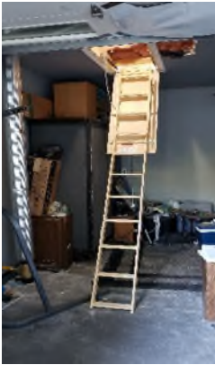
12101 Brewster garage attic ladder
