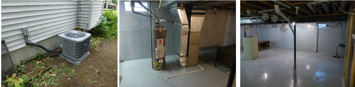
34940 Beacon new air conditioner, furnace and basement after RetroCoat application
