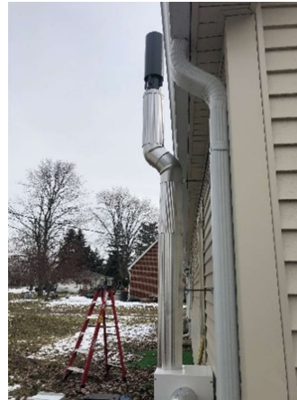
34424 Capitol Mitigation system
