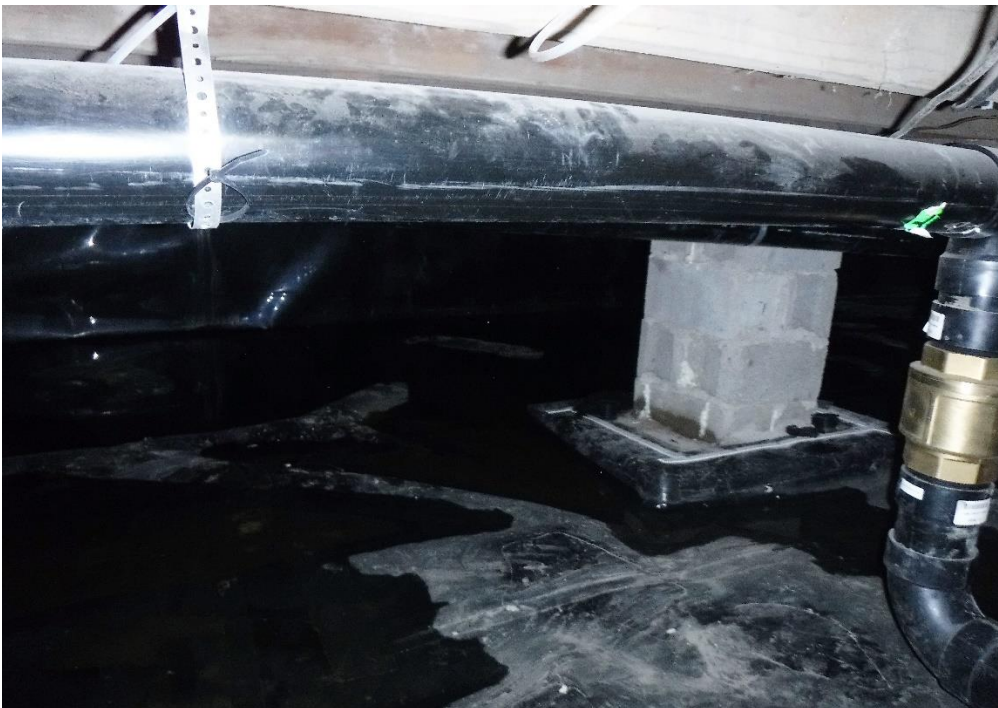
Photo 2 - Standing water on the liner in the crawl space at 34450 Beacon
