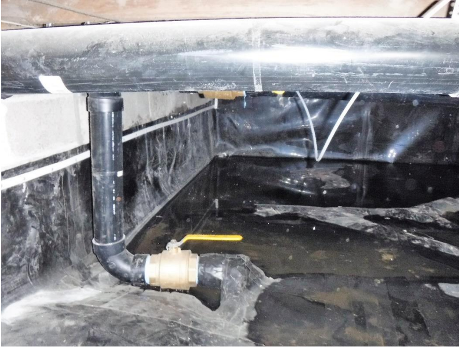
Photo 1 – Standing water on the liner in the crawl space at 34450 Beacon
