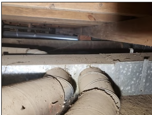
Heating duct without support beam is lying on dirt floor.
