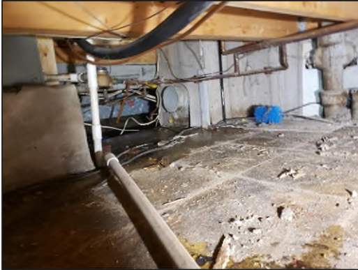
Water meter with multiple leaks
