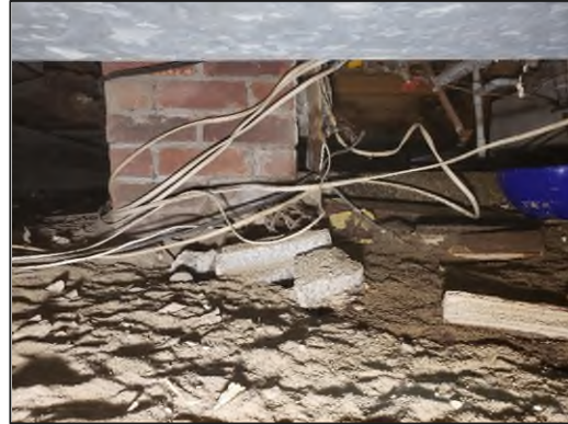
Numerous loose Romex 120V wrapped around a brick pillar.
