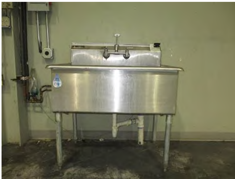
Figure 10. Sink with pipe penetrating the slab.
