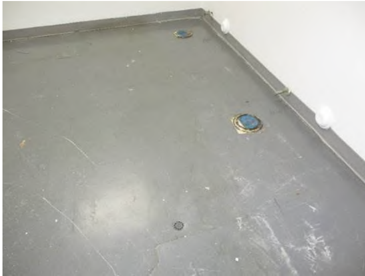
Figure 11. Floor drain and locations where pipes had previously penetrated the slab.
