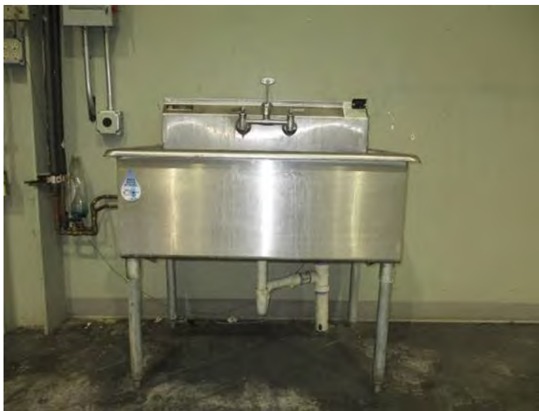
Figure 10. Sink with pipe penetrating the slab.
