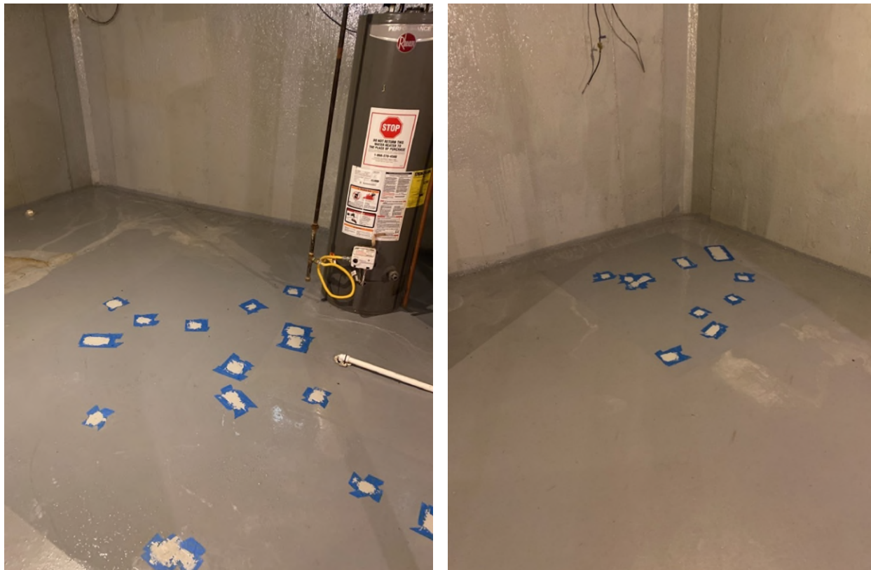
34940 Beacon – Two photographs showing the applied urethane caulk sealing the pinhole depressions in the Retro-Coat®. Photographs taken on June 14, 2024.
