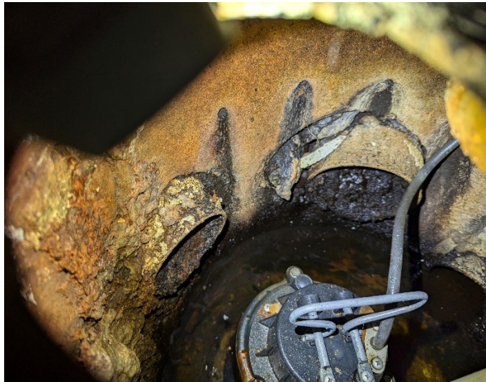
Photograph 2 – The sump basin with clogged inlet pipes.
